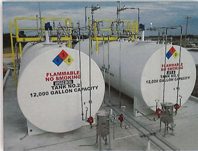
Typical Aboveground Storage Tanks
