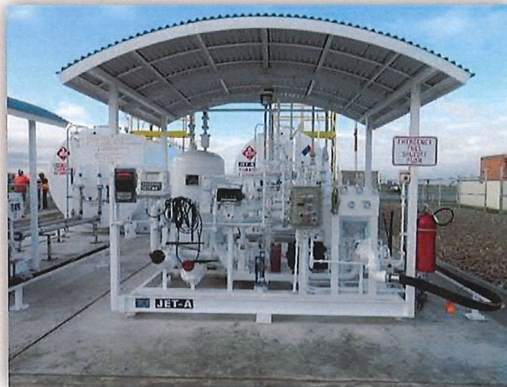
Typical Bulk Loading, Unloading and Recirculation Skid
